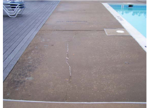
Photo 11 - Cracks in concrete deck
