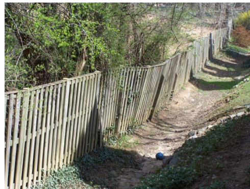
Photo 4 - Damaged wood fence
