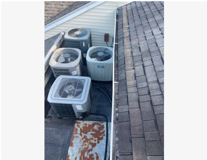
Breezeway Roof With HVAC Units - Overview
