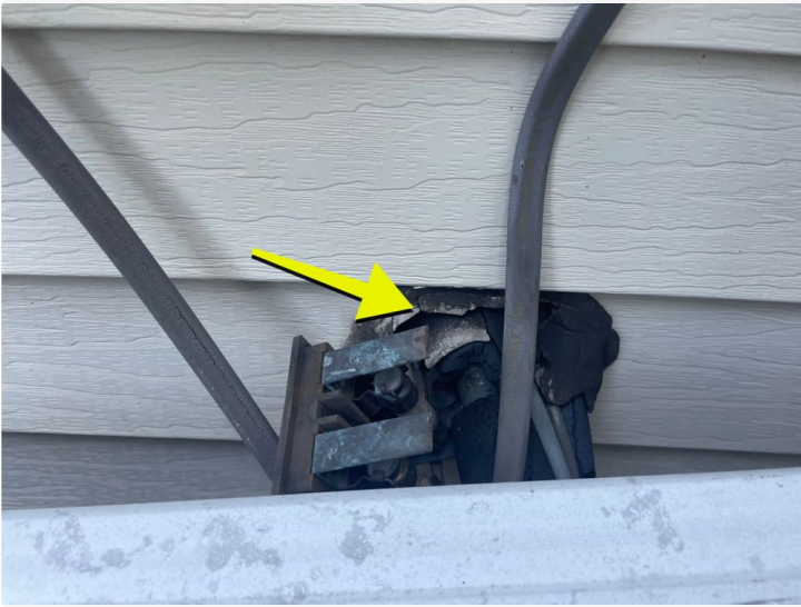
Deteriorated Sealant at electrical housing
