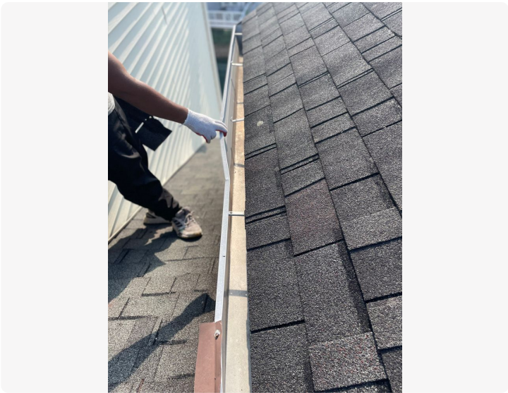
Loose Gutter hangers - As Pictured Below
