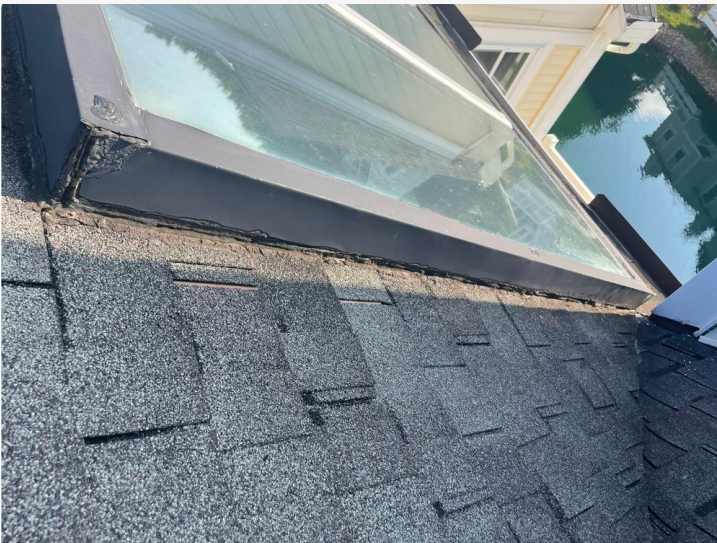
The gaskets are failing and the the glass is separating from the metal frame assembly.
