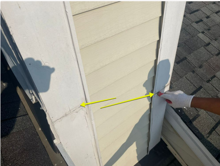
Open Seams at Chimney - As Pictured Below
