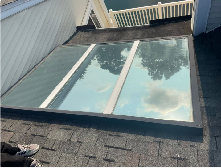
Skylight #1 -The gaskets are failing and the the glass is separating from the metal frame assembly.
