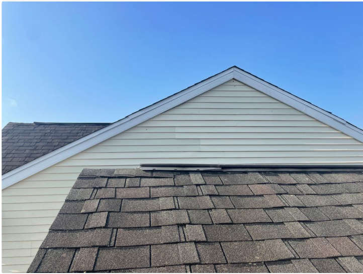
Damaged/Loose Ridge Vents - As Pictured Below
