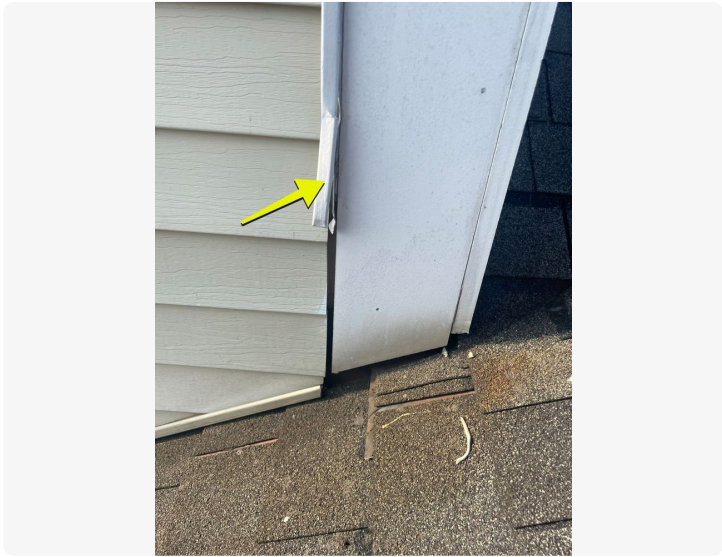
Damaged J Chanel
