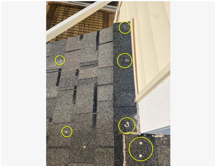
Exposed Nail Heads / Nail pops - As Pictured Below
