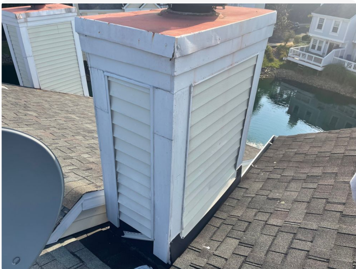
Loose Chimney Cap - As Pictured Below
