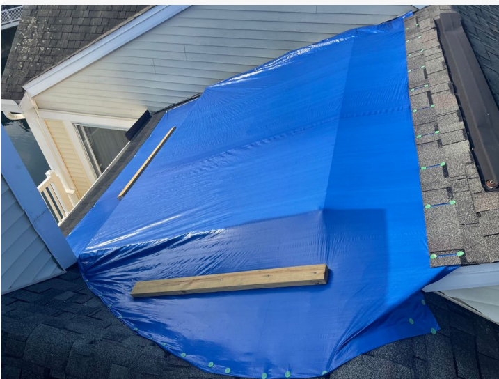
Skylight #2 - Tarped - Needs to be Replaced - As Pictured Below
