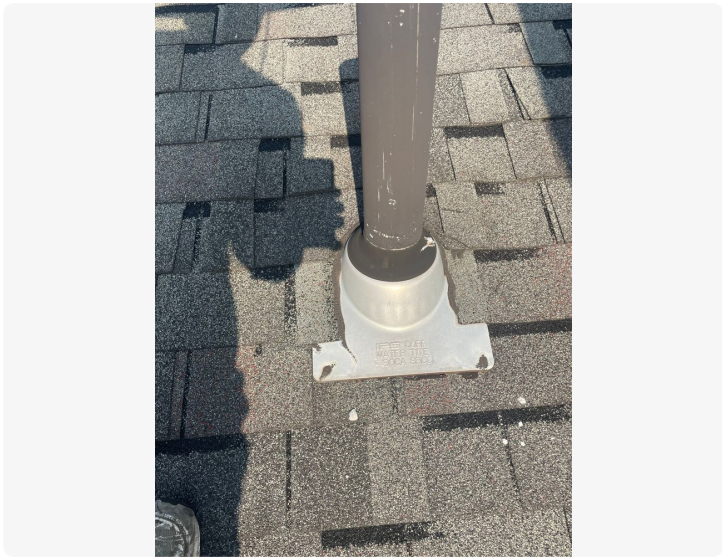
Deteriorated Sealant around Pipes - As Pictured Below
