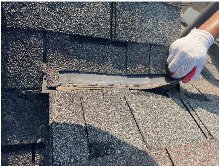
Deteriorated Sealant at flashing
